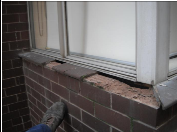
Ph #8659 Level 5 Sill Tiles Missing
