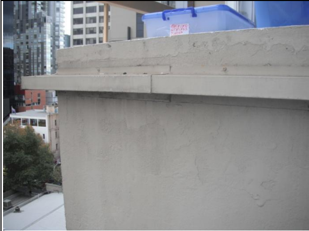
Ph #5188. Level 11 Drummy on top half of wall. 50%
