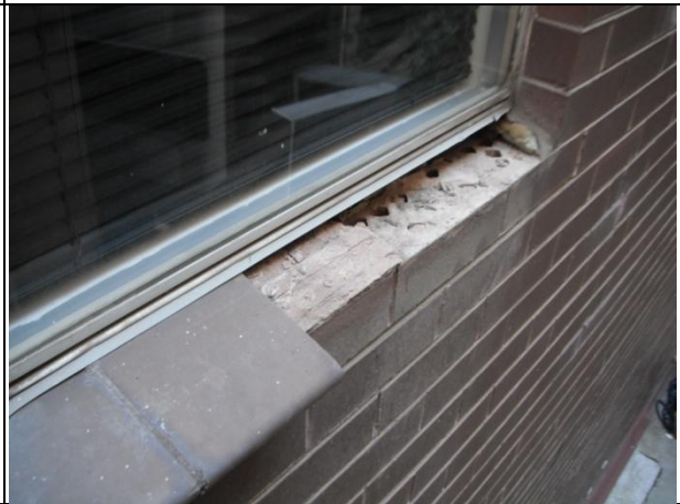
Ph #8660 Level 2 Tiles Missing
