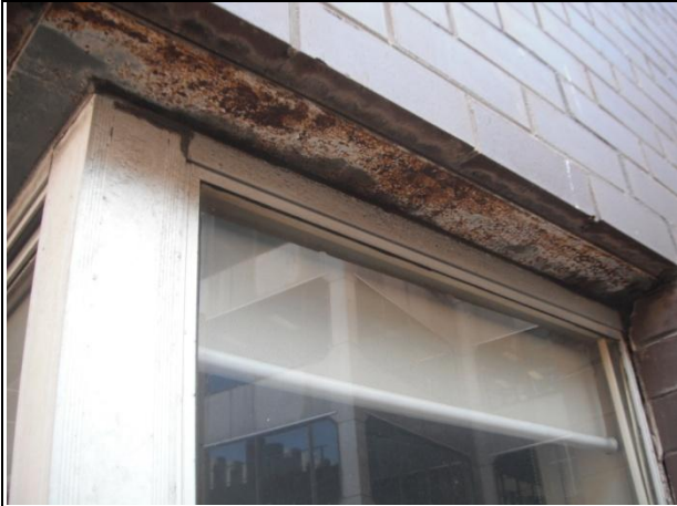
Ph #8657 Level 12 Surface Rust on exposed window Lintel
