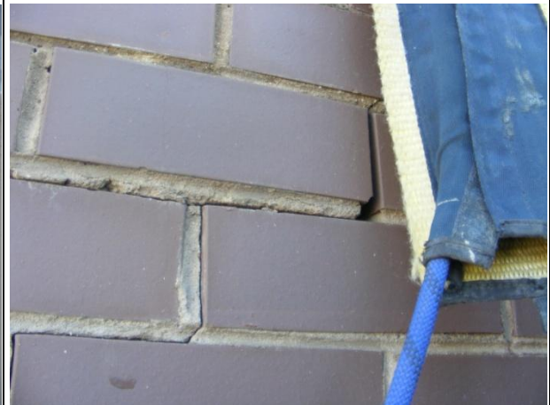
Ph #8746 Level 3 Cog cracking in brickwork
