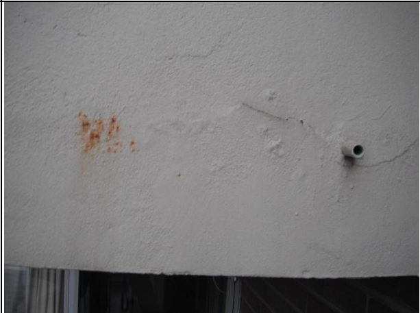
Ph #5525. Significant crack in brickwork
