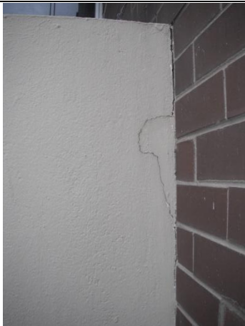
Ph #5194 Level 4 Crack adjoining brickwork
