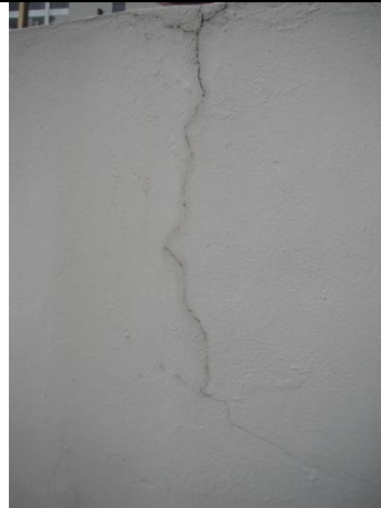
Ph #5189. Level 10 Drummy with significant vertical crack
