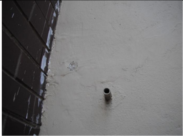
Ph #5473. Level 14 Efflorescence on brickwork. Cracking in render
