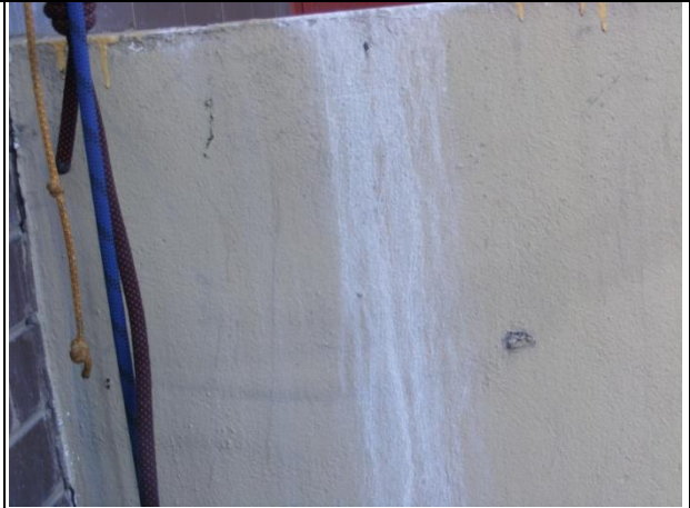
Ph #8752. Level 12. Cracked & Drummy Render. 30%
