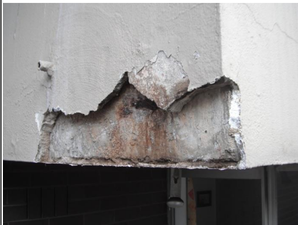
Ph #8664 Level 11 Delaminated Render on corner
