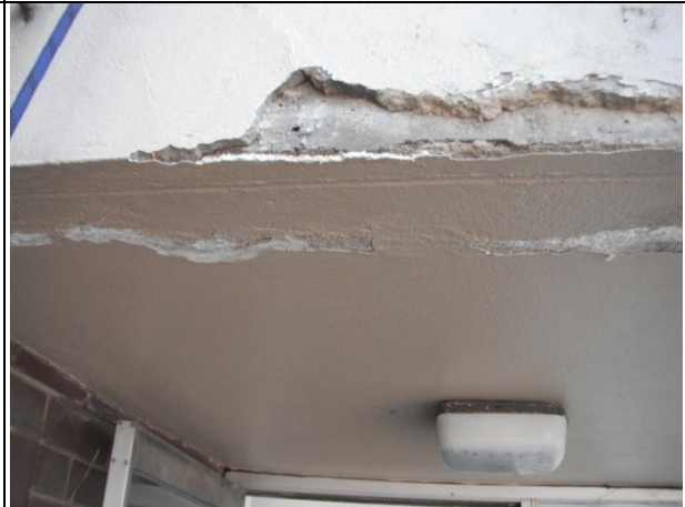
Ph #8662. Level 1 Broken Render Edge. Leak Underneath
