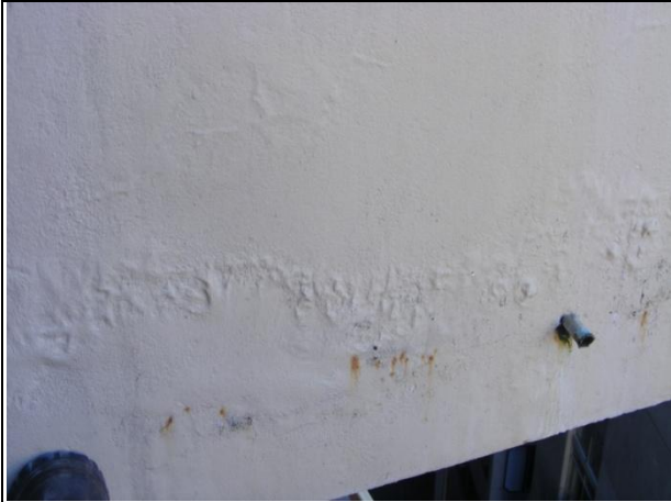
Ph #8751. Level 13 Cracked Render
