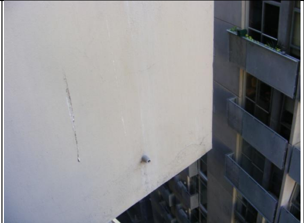
Ph #8753. Level 11 Cracked & Drummy Render. 70%
