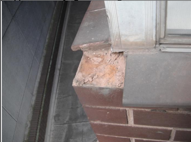
Ph #5491. Level 4 Tile loose. Removed for public safety
