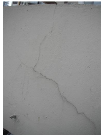
Ph #5192 Level 6. Drummy & Cracked render 30%
