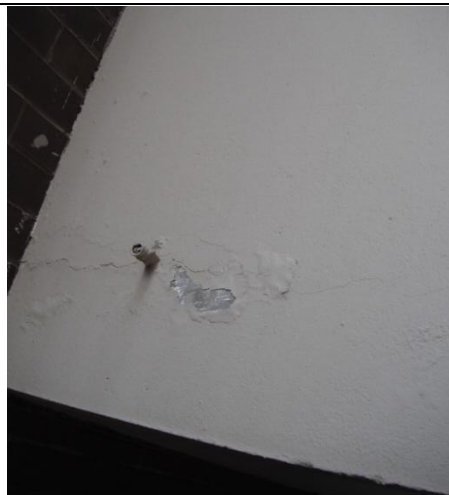
Ph #5480. Level 11. Paint Spalling & Drummy Render
