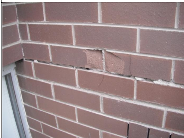
Ph #5527. Level 12 Corroded (Surface) & Lintel Detail
