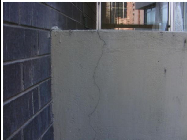
Ph #8757 Level 7 Large Crack in render
