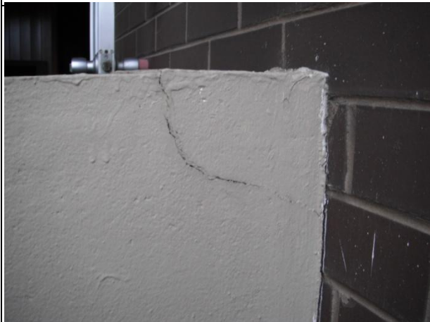
PH #5523 Level 10 Crack adjoining wall
