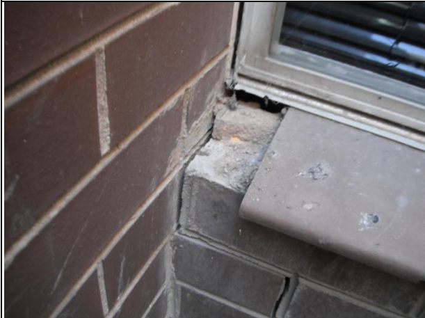
Ph #8661. Level 2 Tile Missing
